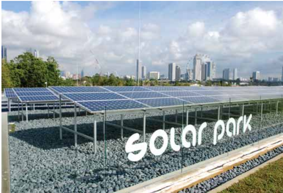
Solar panels at Marina Barrage
